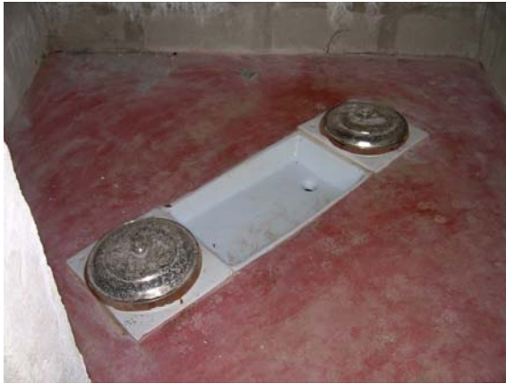
The toilet seen from inside with lids covering the holes to the two chambers and the urine outlet in the middle.
